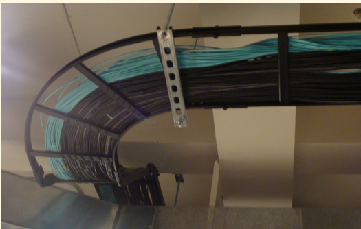
Custom Cable Management
