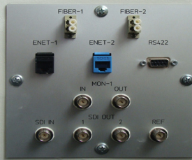
Custom I/O Panel
